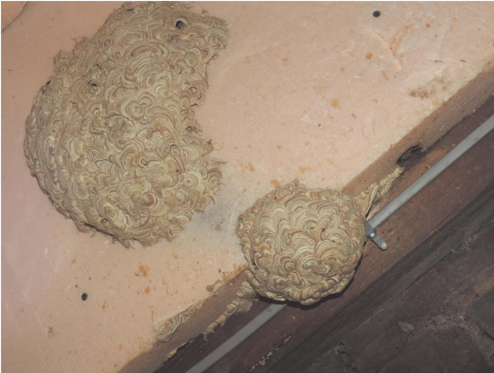
Wasp nest drilled into the roof insulation foam panels
