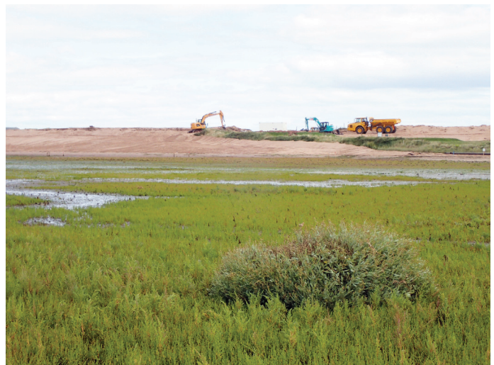
Sea purslane bush where adult Geranomyia bezzii were found at Dawlish Warren National Nature Reserve in August 2017 by Chris Spilling, with major dune re-structuring work in the background. Rob Wolton.
